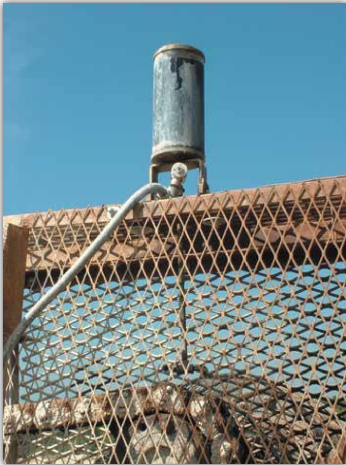
Chain oiler lubricating a chain on a trommel screen
