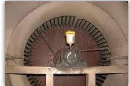
Streamliner V installed on a blower fan
