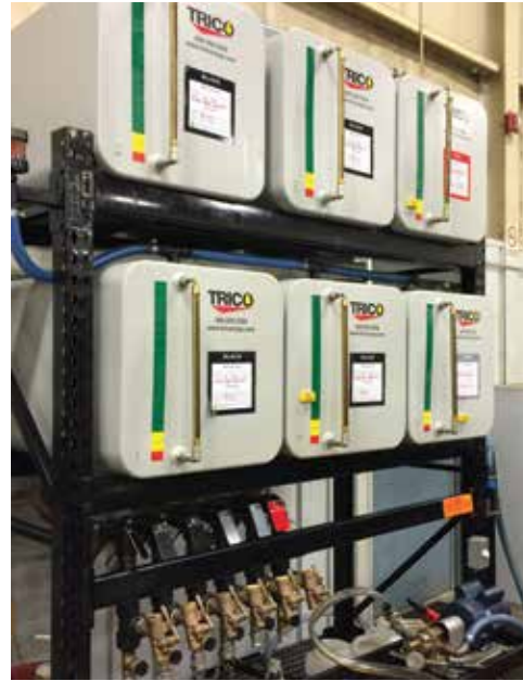
Bulk Oil Storage System - Metal
